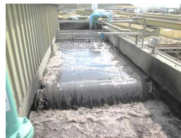
pH Treatment Tank
